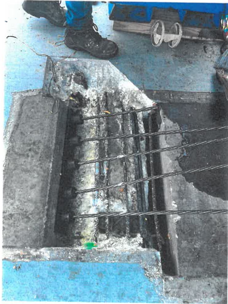
Photograph #1: Post tension anchors near the West slab edge at column line 9A
