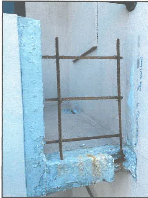
Photograph #1: Typical knee wall repair at the 04 balcony stack requiring supplemental steel
