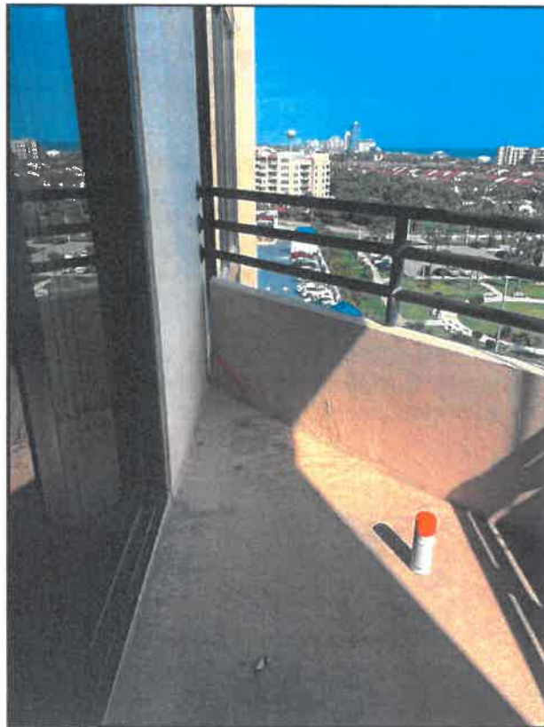
Photograph #2: Damage identified at the balcony of Unit 9A3
