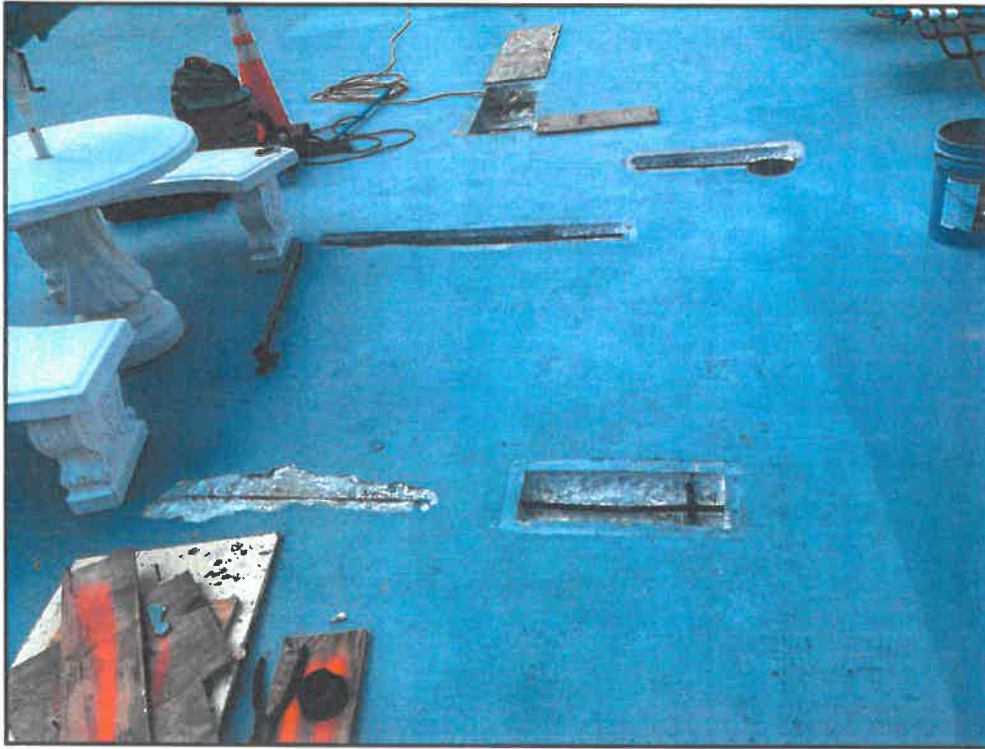
Photograph #3: Accepted and in-progress concrete repairs at the topside of the pool deck
