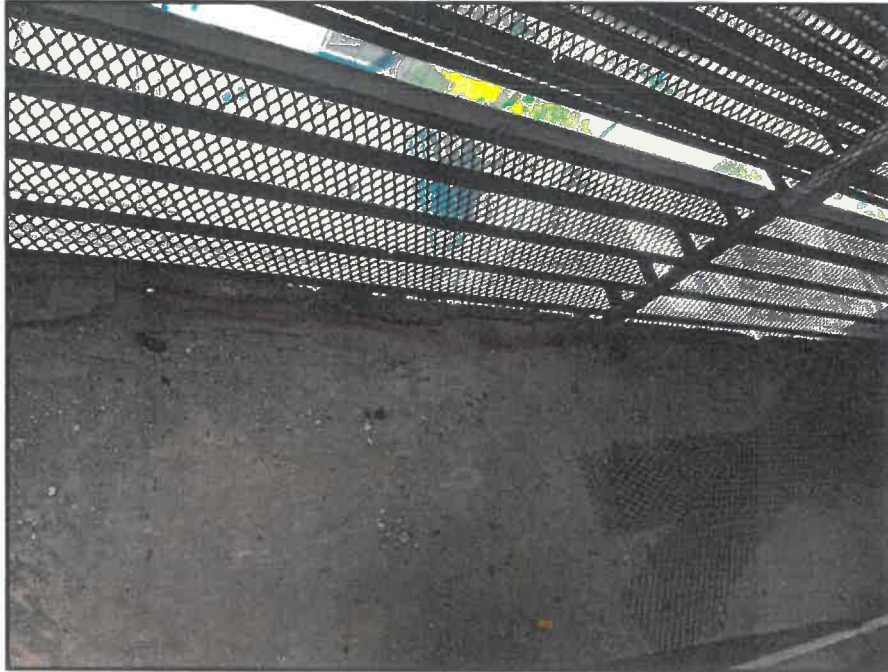
Photograph #1: Damage identified at the 10 th floor slab edge in the A/C closet of the 03/04 stack
